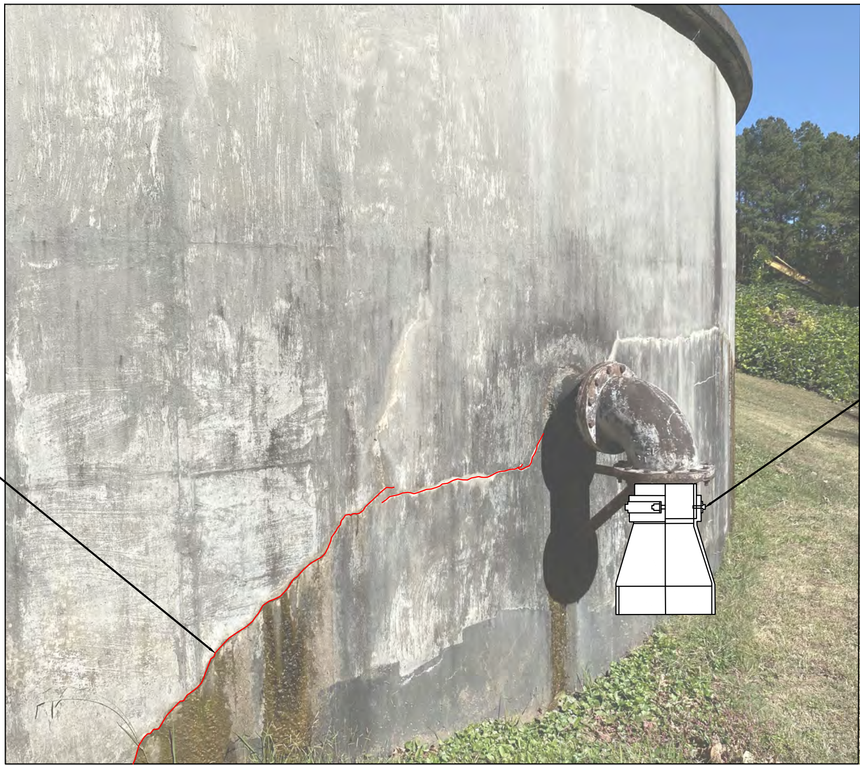
1 FLAPPER VALVE INSTALLATION & CRACK IN CLEARWELL CONCRETE SCALE: N.T.S.
